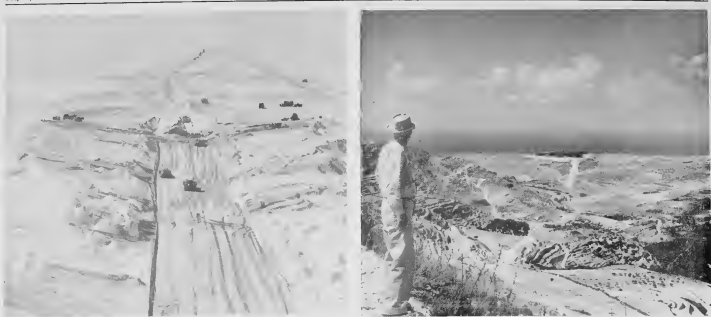
Powerful bulldozers cleared the right-of-way of the trans-Arabia pipeline through a sand dune on the desert near Qaisimah, Saudi Arabia. Many terrain problems were overcome along the course of the pipeline. Near the Mediterranean coast, volcanic boulders had to be blasted out of the way to make way for 30-1/2 inch diameter pipeline. About 60 per cent of the 108-1/2 mile system is buried.
